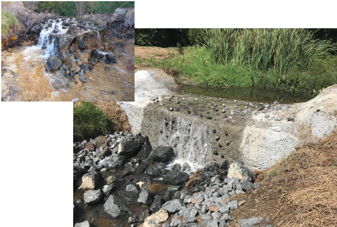
Figure 6-10: Baffled concrete weir in the lower reaches of Puketirini Stream, Waikato. A degraded weir (inset top left) was successfully preventing koi carp, goldfish, perch, rudd and gambusia from accessing upstream habitats whilst allowing the passage of banded and giant kōkopu, and shortfin and longfin eels. To continue protecting native fish populations the weir was remediated in 2018. Credit: Cindy Baker.
