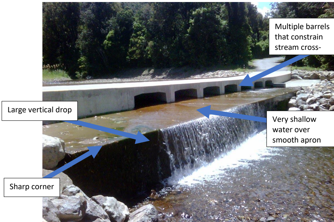
Figure E-18: An example of a drift-deck ford. This is a significant barrier to fish due to the large fall height on the downstream side of the structure. Passage may also be impeded by the sharp corner on the edge of the apron, shallow water, and high water velocities during high flow.
