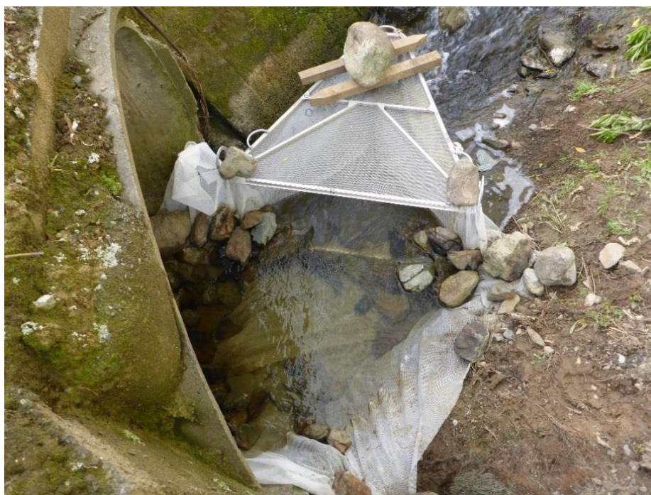
Figure 7-4: Whitebait trap installed at the culvert inlet in Kara Stream.
