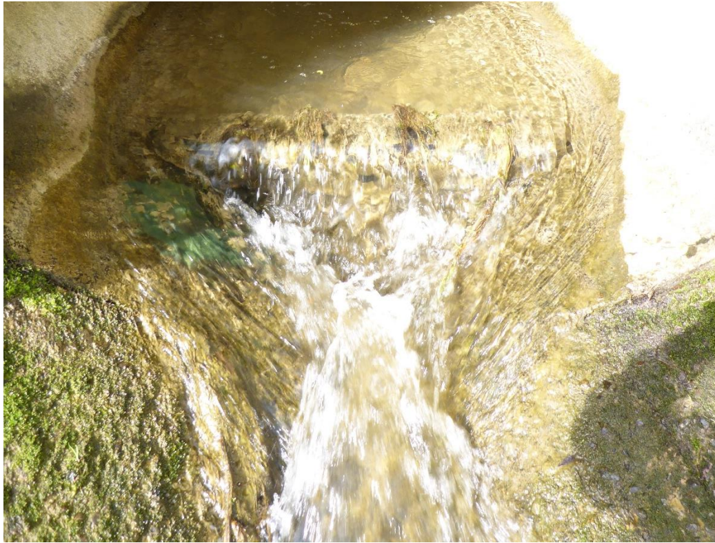
Figure I-6: Weir created by the baffle at the transition point between the culvert outlet and apron.
