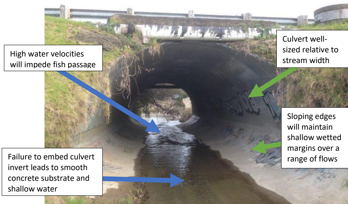
Figure E-23: Culvert well sized relative to stream width, but failure to embed the culvert invert leads to shallow water depths and high water velocity. If this culvert had been embedded so that substrate was retained through the culvert it would have been a good example of how culverts can provide fish passage. Credit: Mark Pennington.
