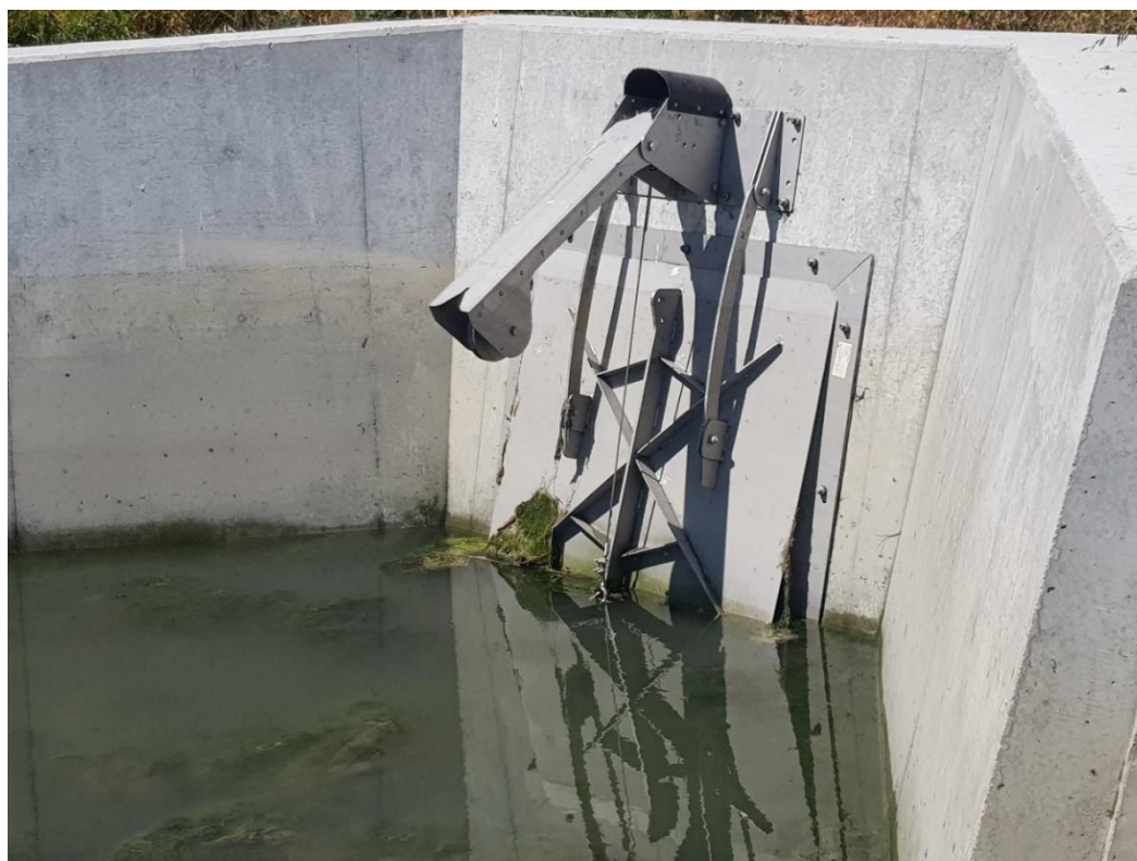
Figure 4-19: Example of a self-regulating tide gate installed in Canterbury. The counter weight system holds the tide gate open for longer on the incoming tide. The system can be calibrated to manage the magnitude and duration of the opening to best coincide with critical migration periods, e.g., the incoming tide for whitebait and eelers.
