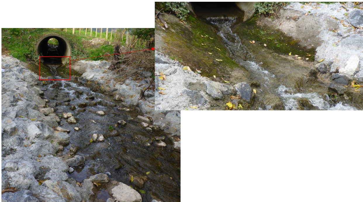
Figure I-1: Remediated culvert on Kara Stream, Upper Kingston Road. Inset shows the unmodified culvert apron.
