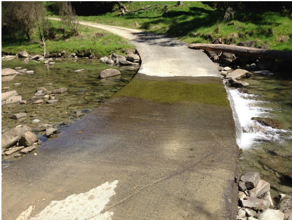
Figure 4-16: Raised roadway ford crossing. The vertical drop on the downstream side will block fish movements. Shallow water depth and elevated water velocities across the ford pavement can also impede movements.
