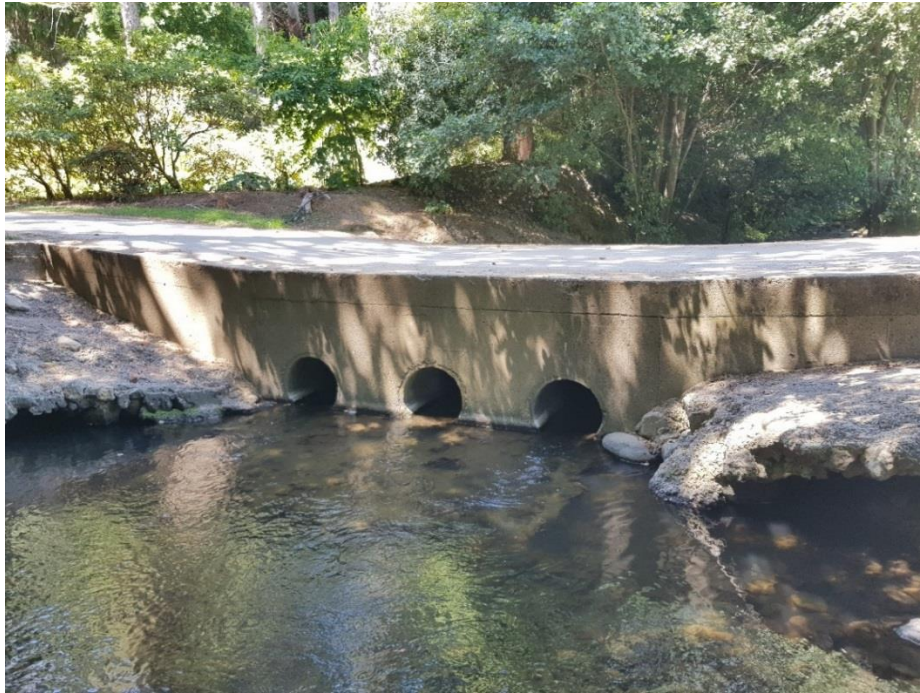
Figure 4-17: Raised roadway ford crossing with culverts. At low flows water passes through the culverts in the ford, rather than over the roadway. The small culverts used in this ford severely constrict the river channel and will result in accelerated water velocities through the culvert barrel that may be impassable to fish.
