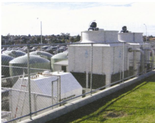
On-site green tanks
