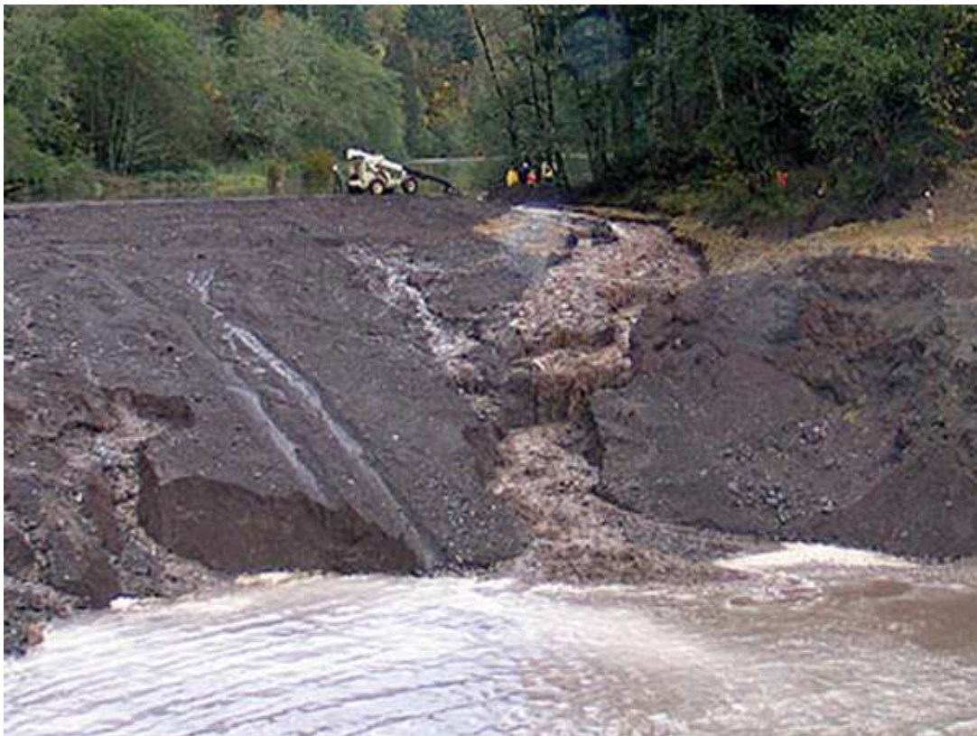
Cutting a breach in the temporary earth dam in the background of the previous two photos.
