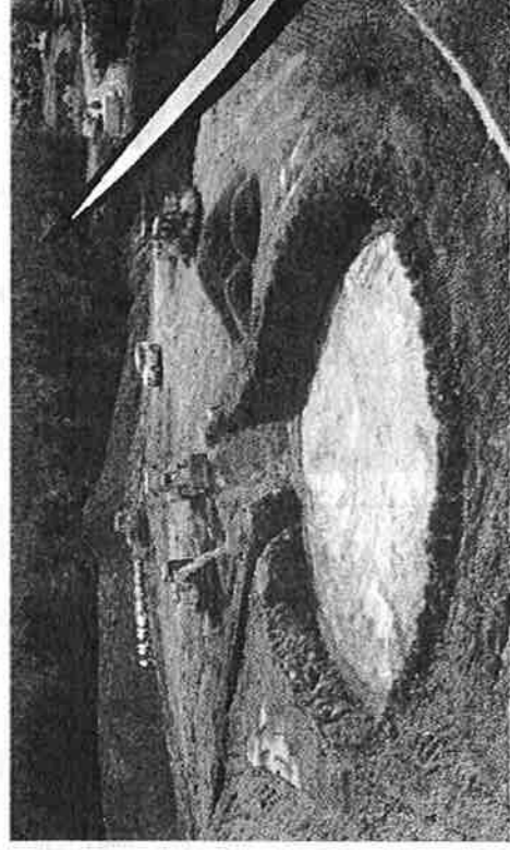
SITE clearance for one windmill. Is this PNCC's idea of an eco park?
