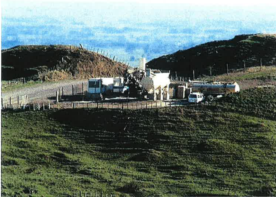
Photograph 5 : Typical concrete batching plant
