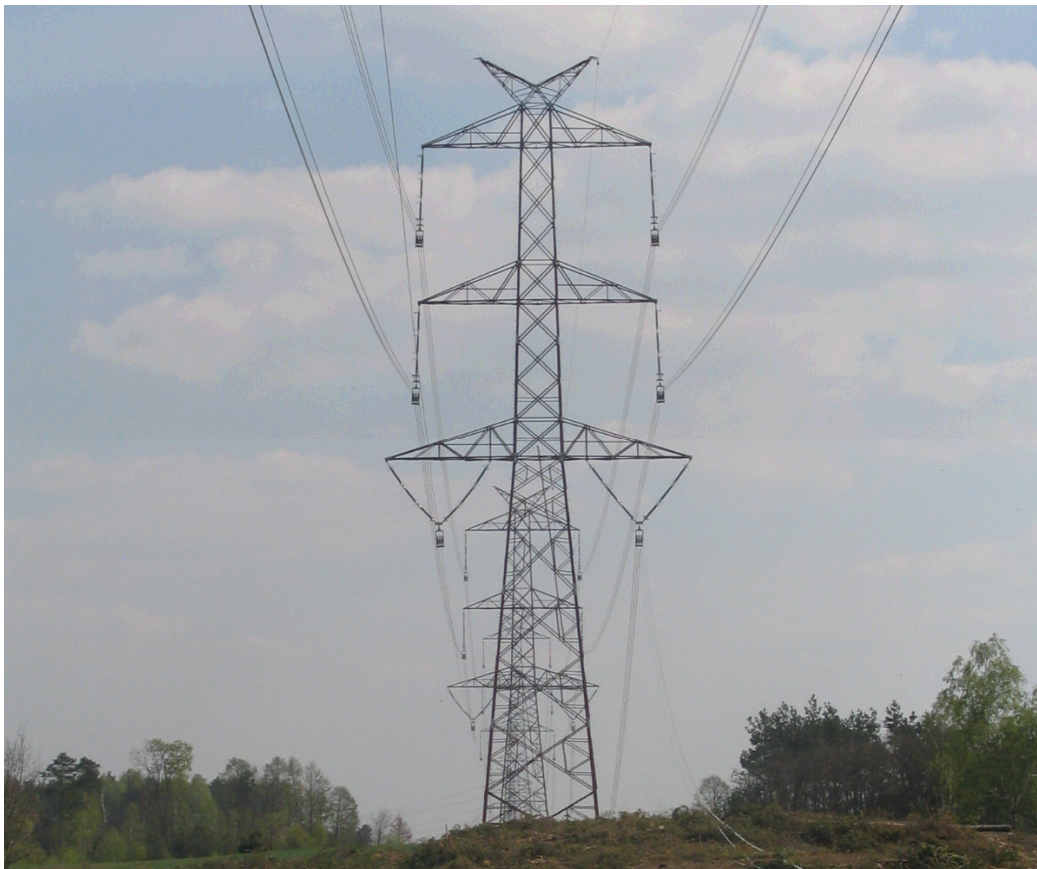
Figure 8 Photo of Typical V String Insulator Arrangement (Bottom Phases)
