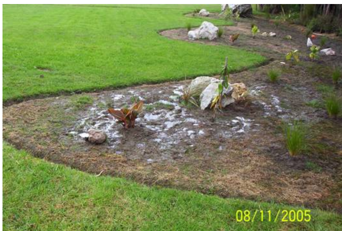
Figure 3: A failed system with sewage effluent discharging onto a flower bed
