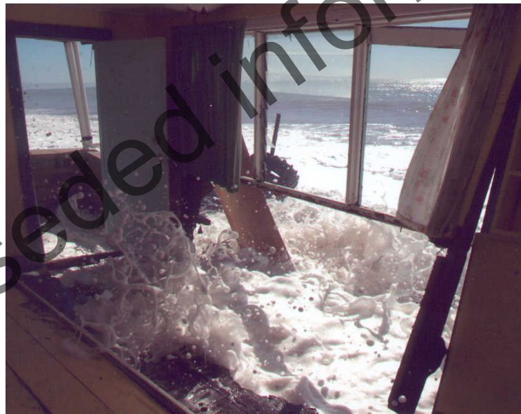
Figure A3.3: Damage caused to a coastal property at Haumoana (Hawke's Bay) by waves overtopping the gravel barrier in the Easter storm of 3–4 April 2002, assisted by high perigeon-spring tides. [Source: Hawkes Bay Regional Council].
